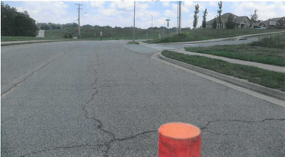
Figure 37 - Eastbound Approach with 2-Foot Object in View, 340 Feet Away (Wide Angle Photo)
